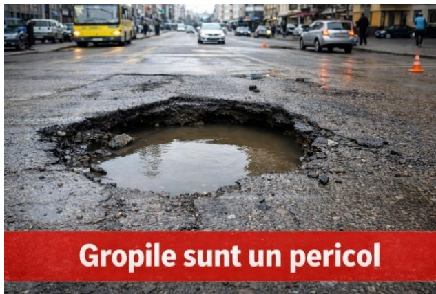
1. Pothole in major intersection
